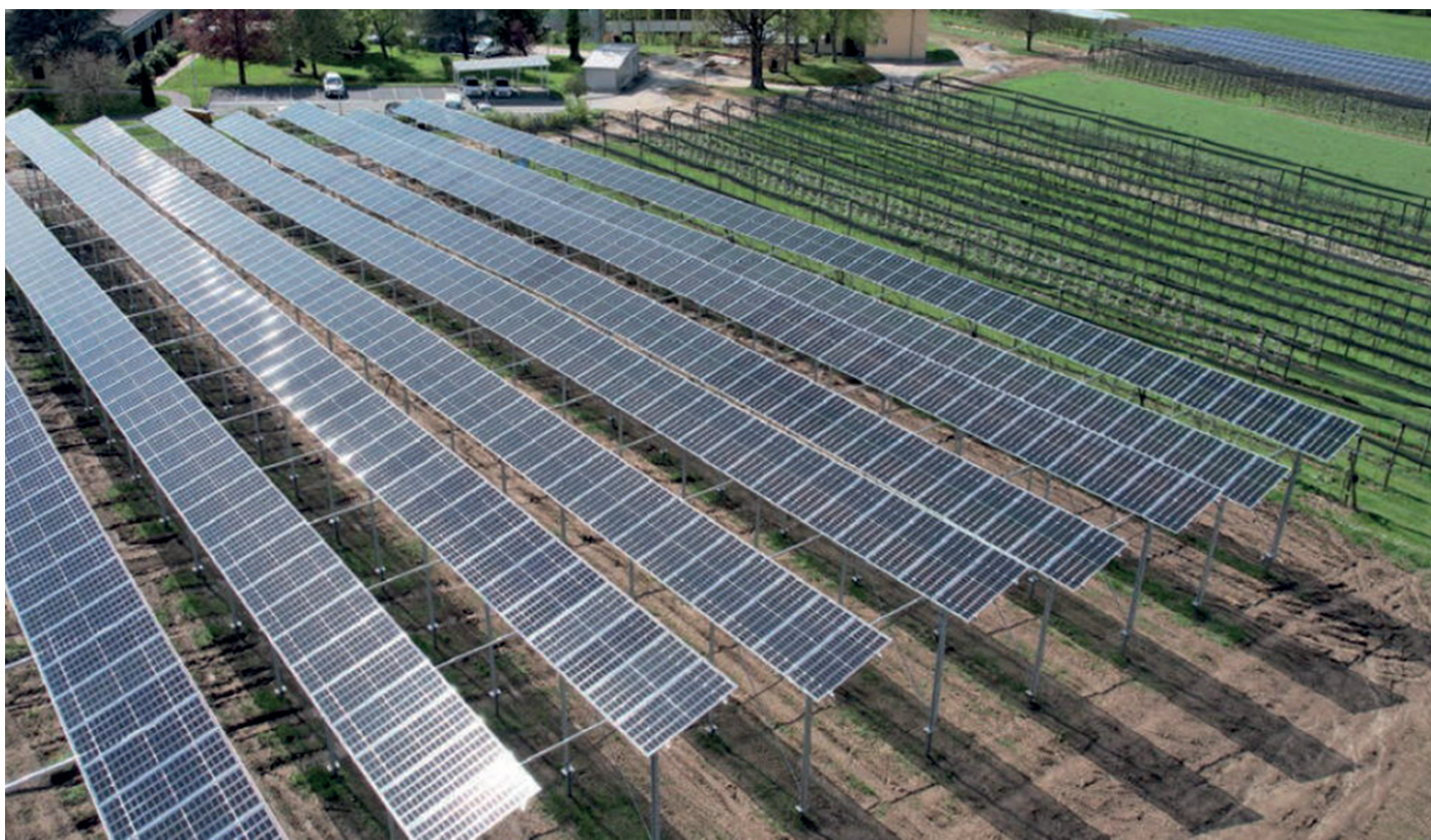
Figure 20 Comparative aerial view of the installed system of APV system Haidegg
