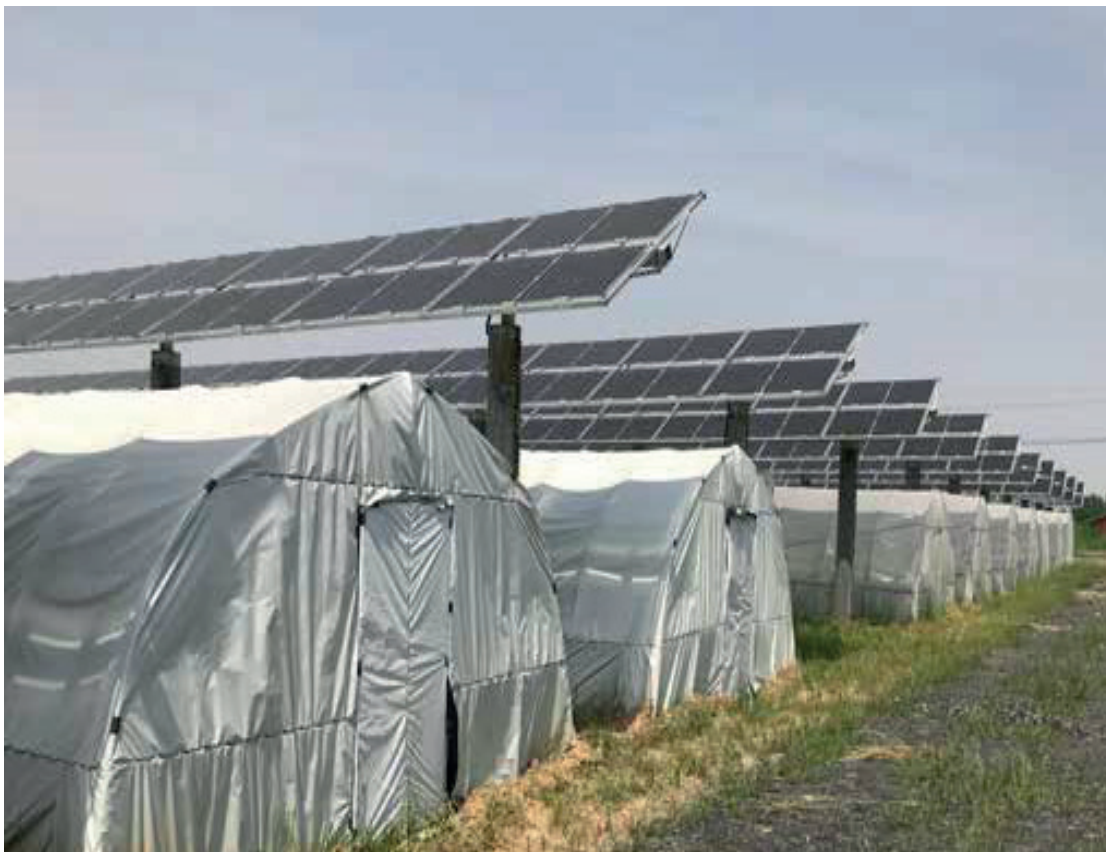
Figure 2 PV modules above a foil tunnel
