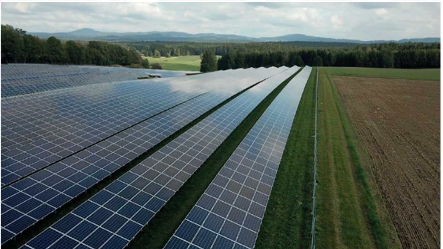
Figure 31. Kozani solar park
