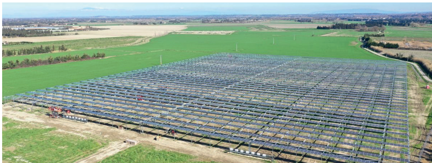
Figure 24 Saint-Etienne-du-Grès agrivoltaic system
